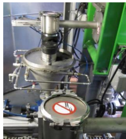
Figure 7: Station de dosage de CAP
